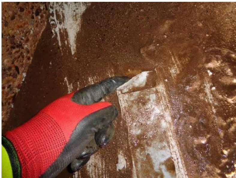
Figure 46 – Sediments in Bourne Vale Contact tank
