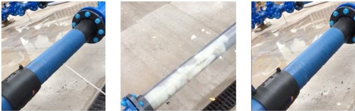
How TALR works to fix background leaks that might not otherwise be cost effective to locate and fix.
