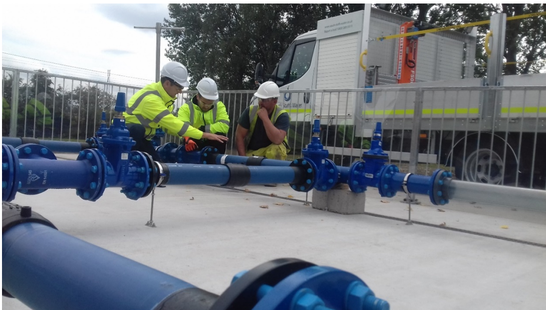
Our TALR test facility at our Trent Valley site.
